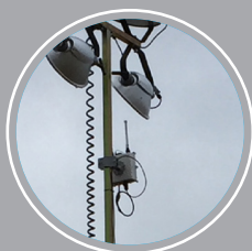
DSRC ROAD SIDE UNITS
